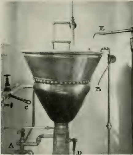
Fig. 9. Jordan Hospital. Sterilizing slop sink.
